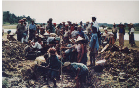
Tens of thousands of people were forced by the Burmese military to help build the Yadana-Yetagun gas pipelines.
